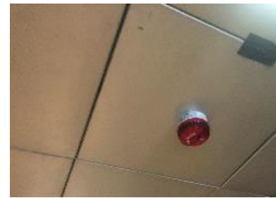
Visual fire alarm system
