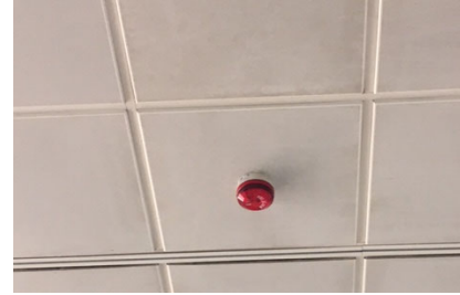
Visual fire alarm system
