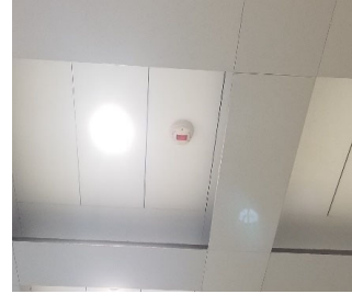
Visual fire alarm system
