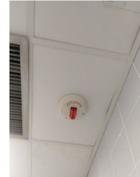
Visual fire alarm system
