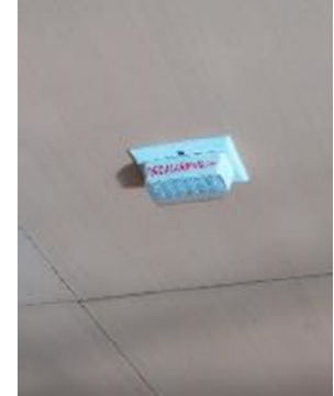
Visual fire alarm system
