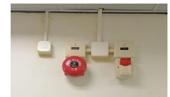
Visual fire alarm system
