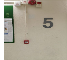
Visual fire alarm system
