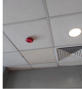
Visual fire alarm system
